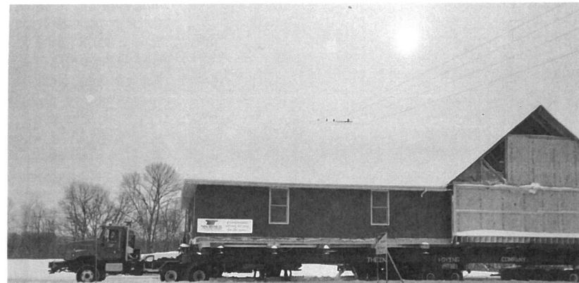
Moving and adding on Of New addition: Fellowship hall, Foyer, Drive Thru.
